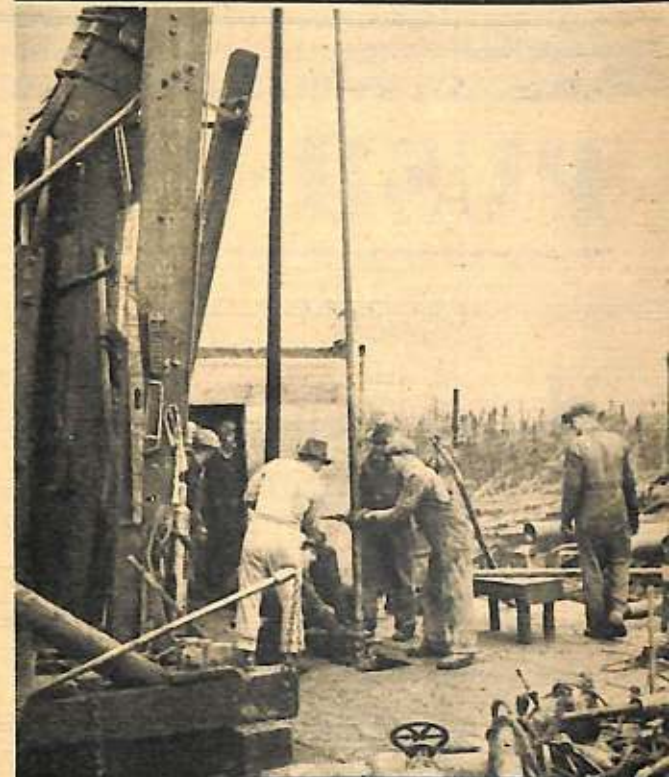
Army Engineers supervise lowering of production pipe on a well of the Canol project at Norman Wells. From there the oil is piped 577 miles to Whitehorse.
