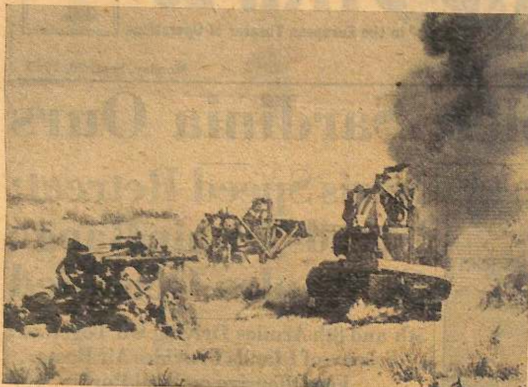
Germans scarcely had been cleared from the Salerno area before U.S. Engineer units were rebuilding communication lines. Two enemy vehicles still burn as a U.S. bulldozer cuts a road through the sand dunes.
